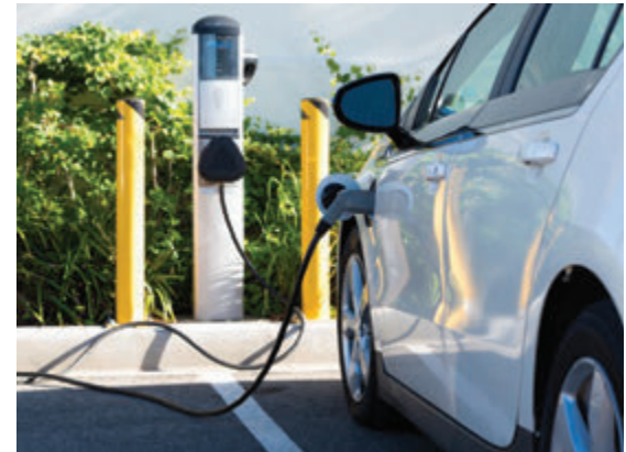
EV charging infrastructure
